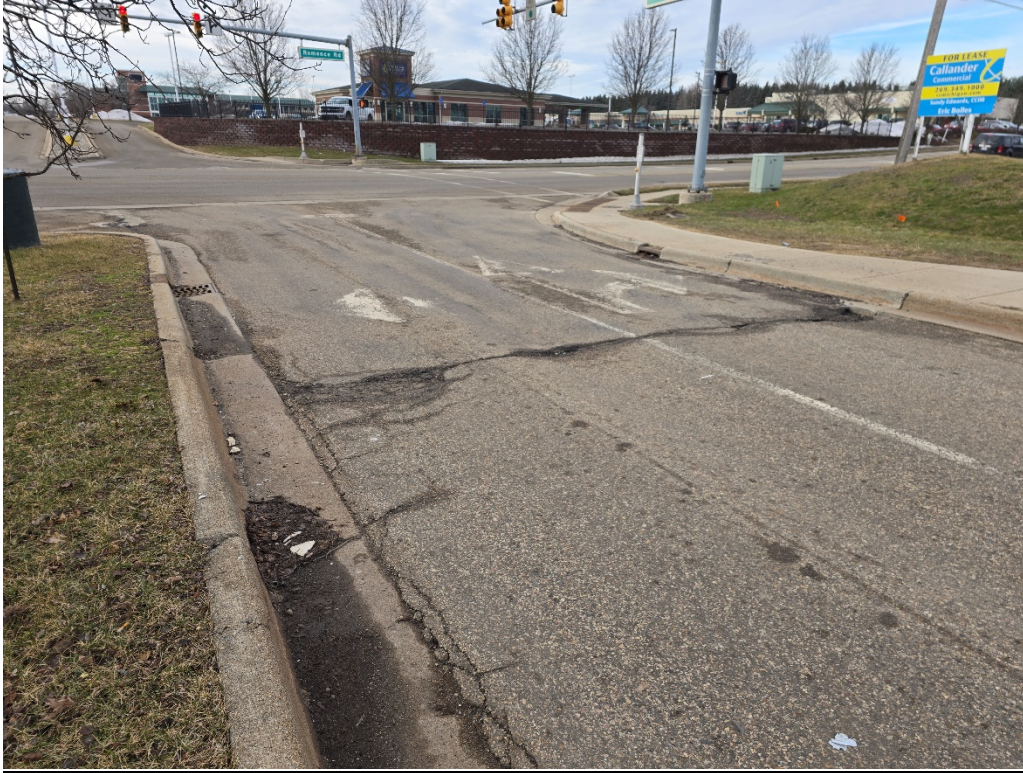
Figure 8: Sears Drive-Romence Road intersection facing south; severe distortion/rutting in pavement surface
