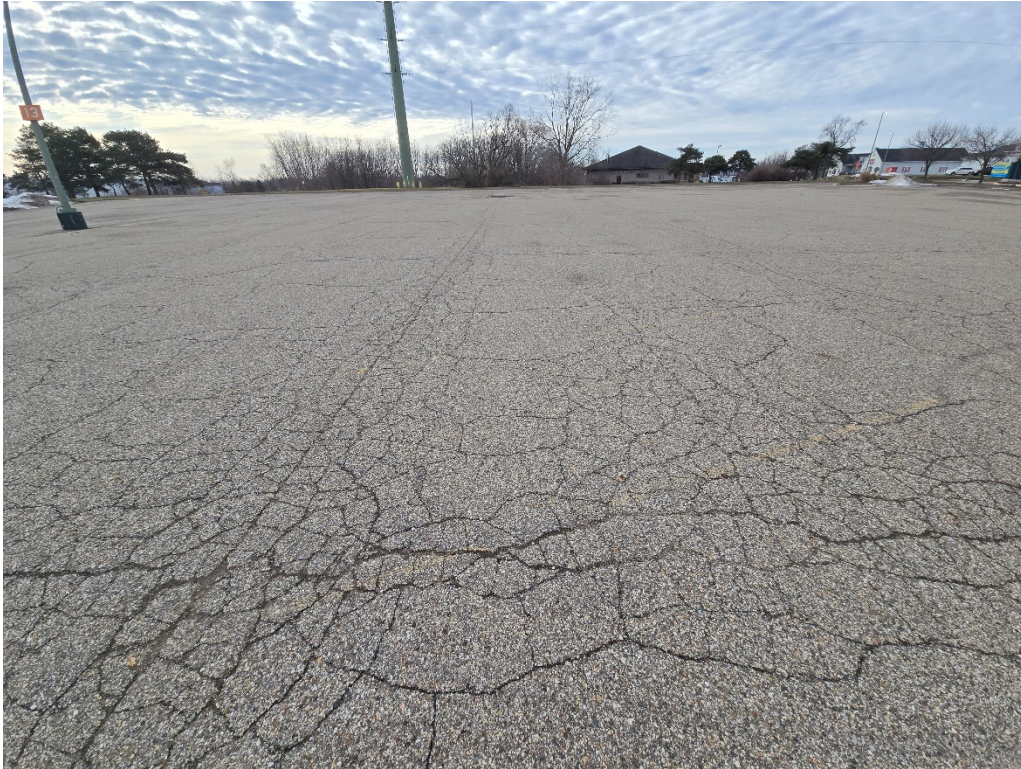
Figure 4: View of parking lot facing south from building; extensive block and alligator cracking observed.
