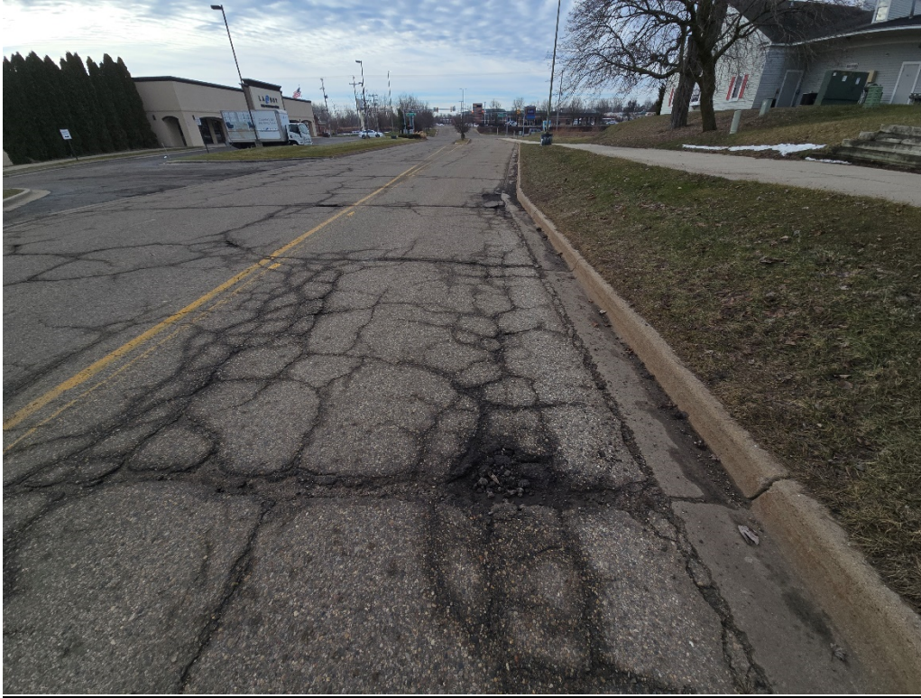
Figure 10: Sears Drive facing south towards Romence; Severe cracking and raveling with potholes
