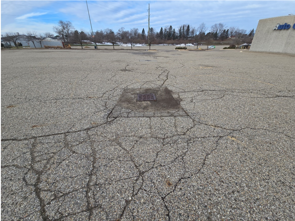
Figure 6: Parking lot facing west, south of building; evidence of surface ponding due to pavement failure around structure.
