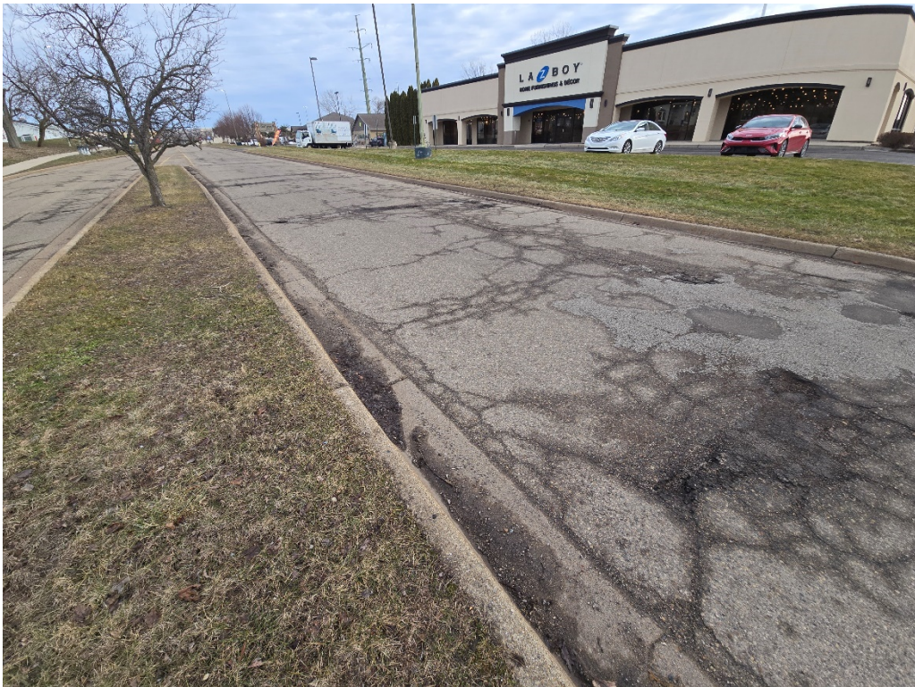
Figure 9: Sears Drive facing North; Severe cracking and raveling with potholes and poor patches
