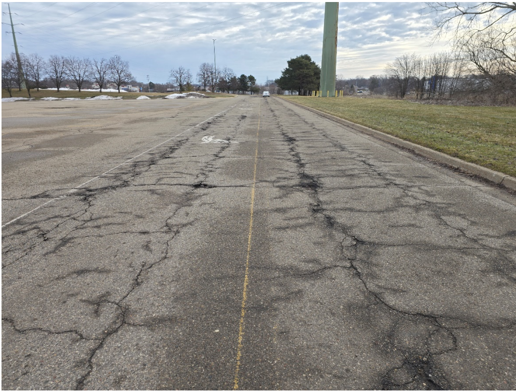
Figure 13: Mall Ring Road East of Sears Drive; Severe cracking and potholes in wheel paths
