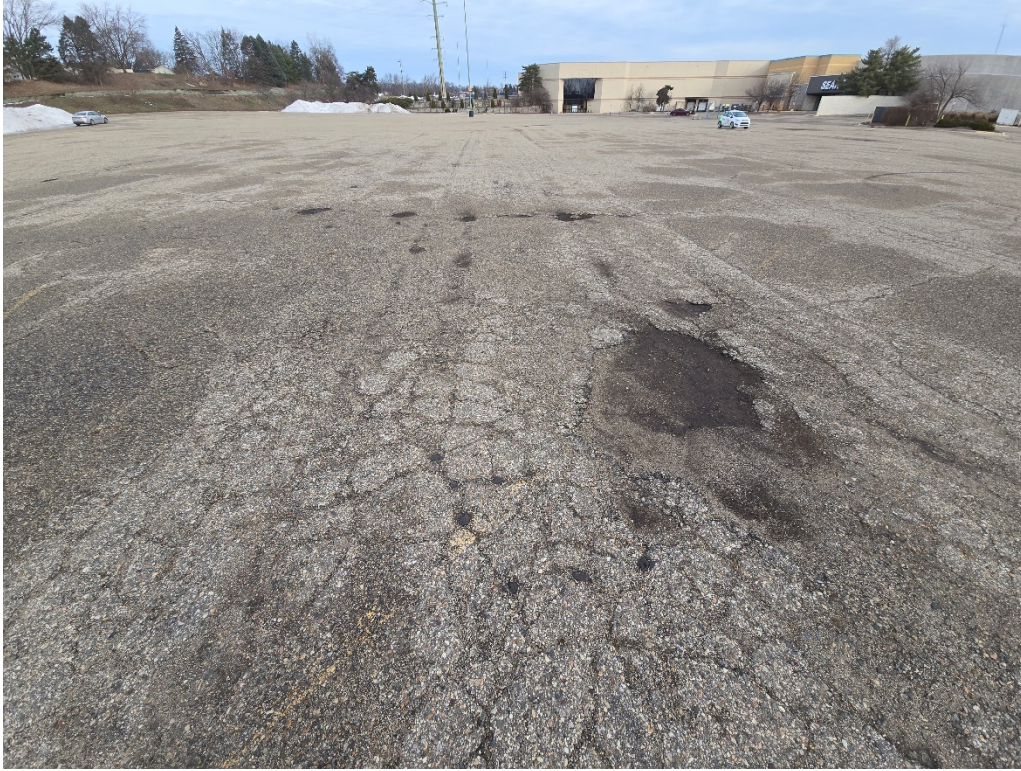
Figure 3: W-SW Parking Lot looking north; extensive block and alligator cracking with large potholes/missing pavement areas.
