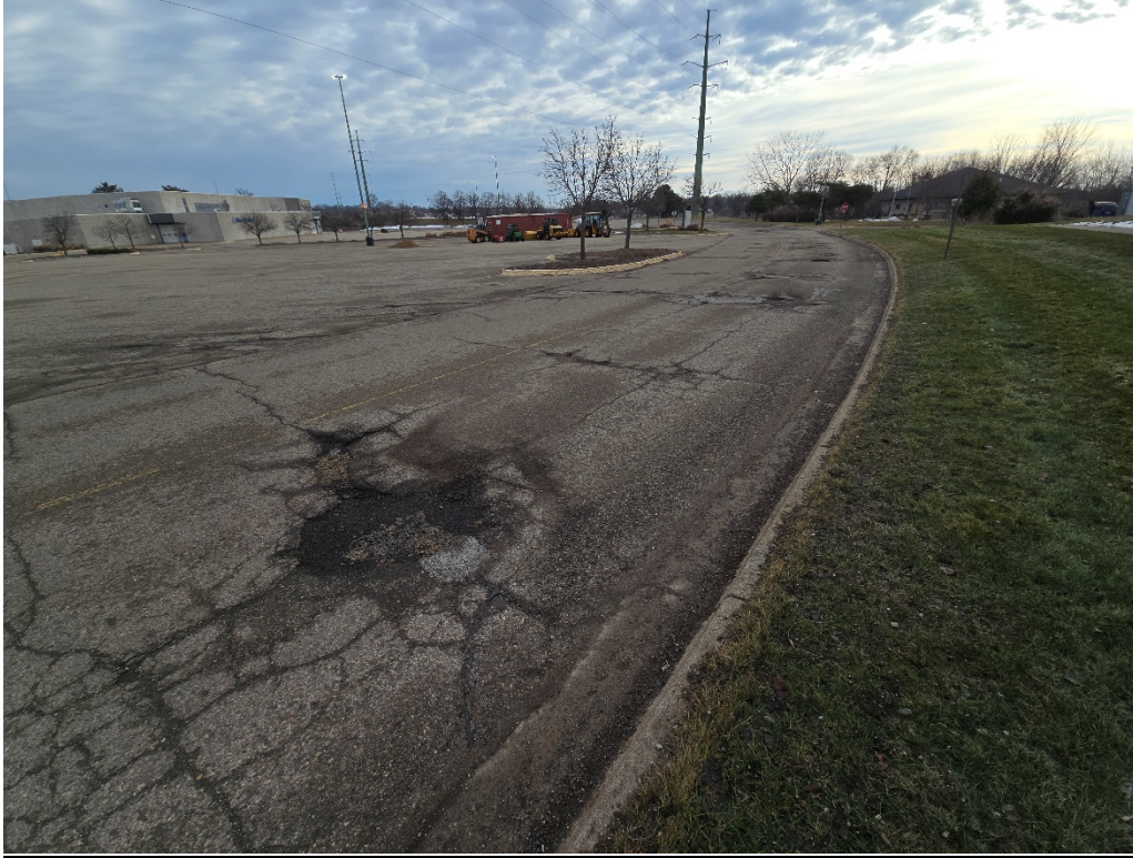
Figure 12: View of Ring Road facing E-NE, west of Sears Drive; severe cracking, raveling present with potholes and poor patches.
