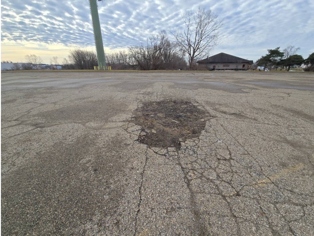
Figure 5: Large pothole south of building with open and raveled block cracks
