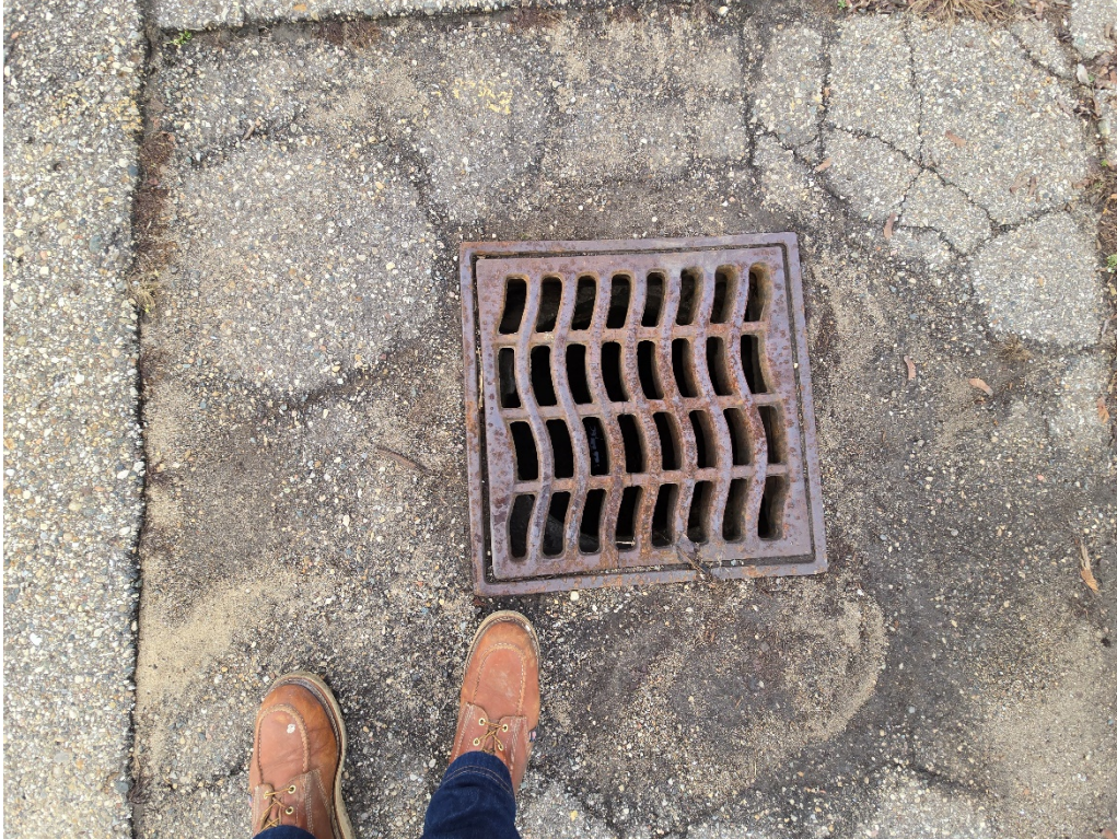
Figure 7: South of building; patch around structure in very poor condition, casting grate nearly split in half.
