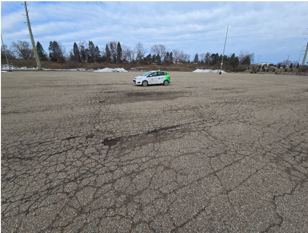
Figure 2: View of parking lot facing W-SW from building; extensive block and alligator cracking present with potholes.
