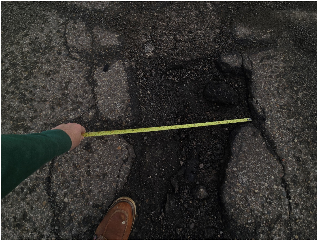
Figure 11: Pothole on Ring Road approximately 2-feet across
